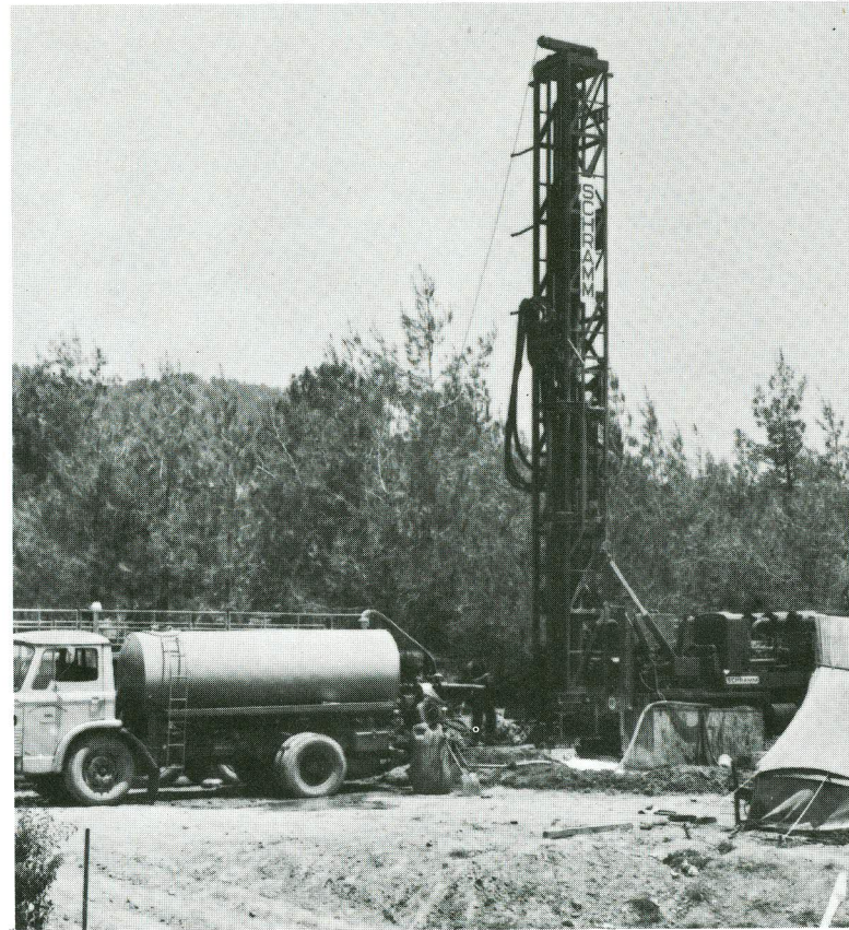
A total area of about 300 hectares will be irrigated in the Project region from some 20 boreholes drilled with heavy rotary drills.
