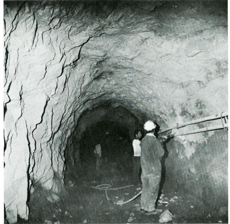
Construction of Xyliatos dam is well under way. Construction of a 110 metres long diversion tunnel (photo) and of the coffer dam has been completed while all other related activities are in full progress with the aim impounding to be effected early in 1982 and scheme completion by the end of the same year. The dam has a capacity of 1.3 million c.m. and will irrigate 300 hectares.
